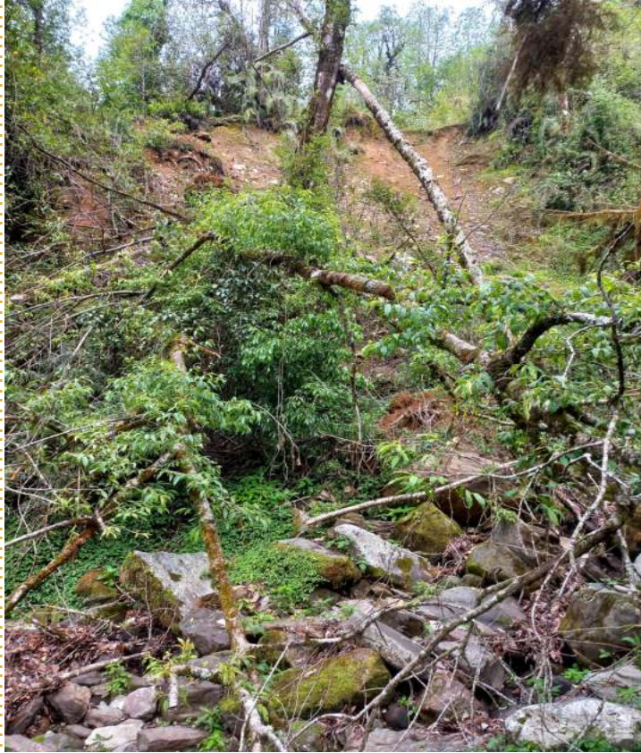
Slope failure near streams
